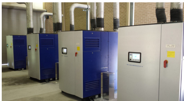
The Shortland compressor room
